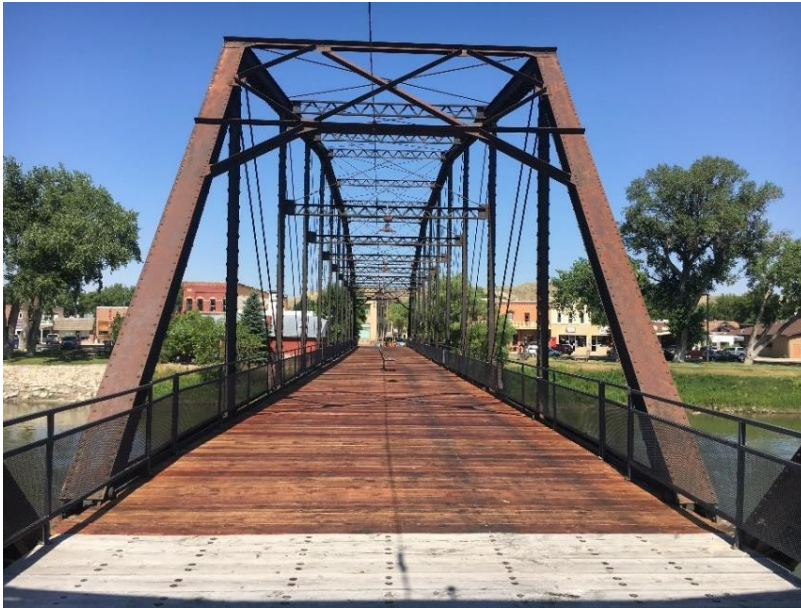
View of similar completed timber deck replacement on the historic Fort Benton Bridge (2017)
