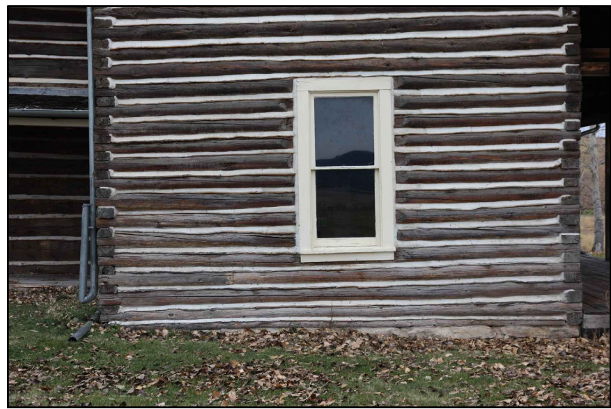
CHIEF'S HOUSE SOUTHWEST CORNER WITH SETTLING
