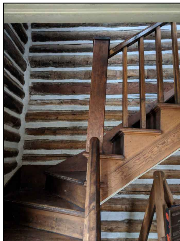
CHIEF'S HOUSE SETTLING AT INTERIOR SOUTHWEST CORNER
