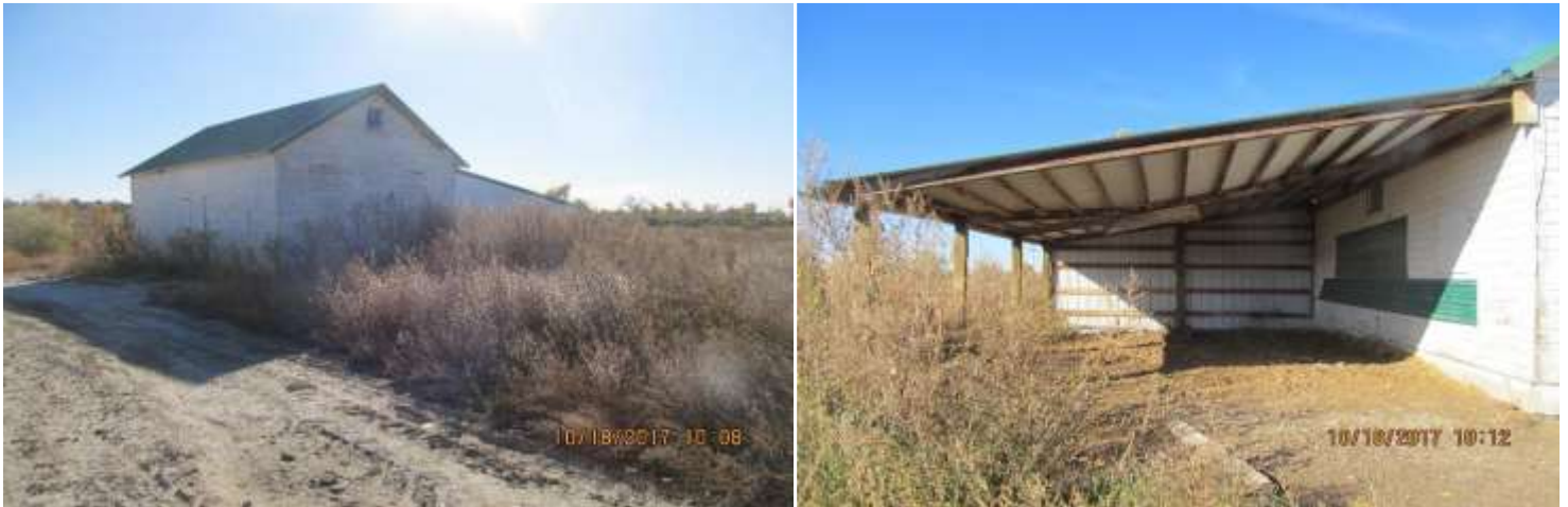
Figure 2. (a) Building to be repaired and improved. (b) lean-to attached to building two. Also, to be repaired and improved.
