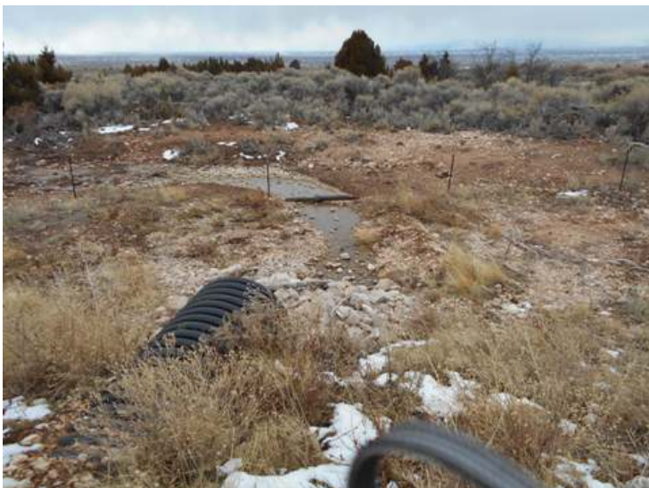
Figure 4: Water downstream of leaking embankment.
