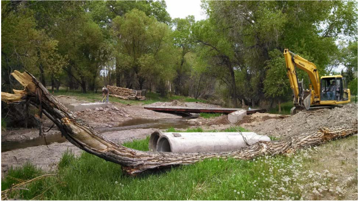
Figure 1: New bridge over Spokane Creek under construction. Fencing will be on the left bank in the picture.
