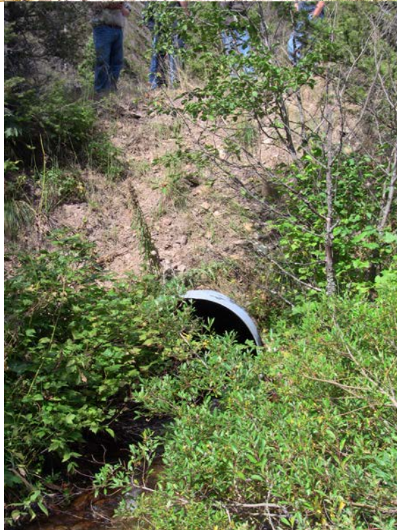
Photos 1-2: Existing outlet and inlet on stream crossing structure near stream-mile 0.1 on Gleason Creek.
