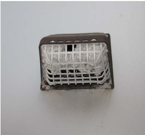
Figure 4 Note the potentially dangerous lint build up on this screened dryer vent.
