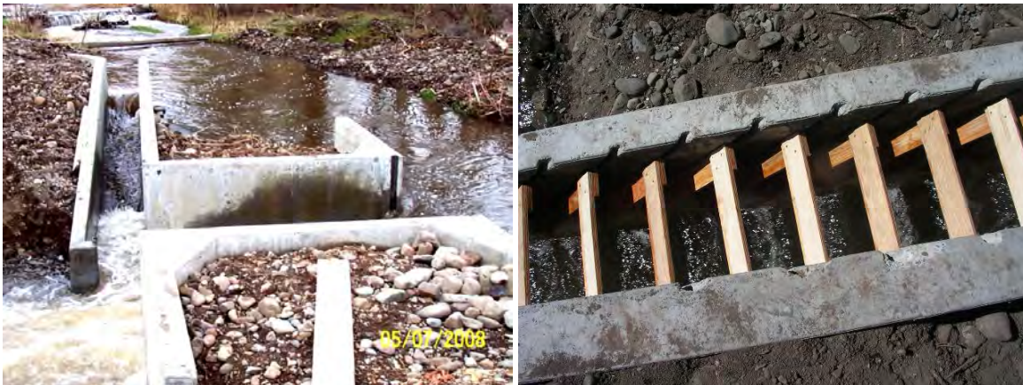
FIGURE 101. NEWLY CONSTRUCTED FISH LADDER (L) AND WOODEN BAFFLES (R) ON SOUTH FORK FRIDLEY CREEK
