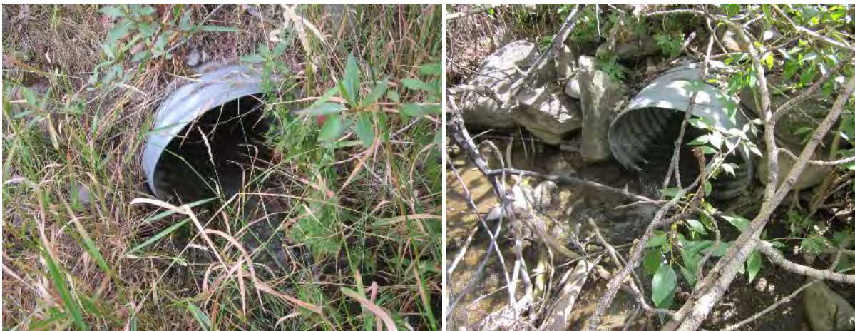
FIGURE 57. INLET OF PIPE THAT PASSES THE UNNAMED SPRING CREEK UNDER THE CORRALS ADJACENT TO ELK CREEK (L) AND OUTLET OF PIPE (R).
