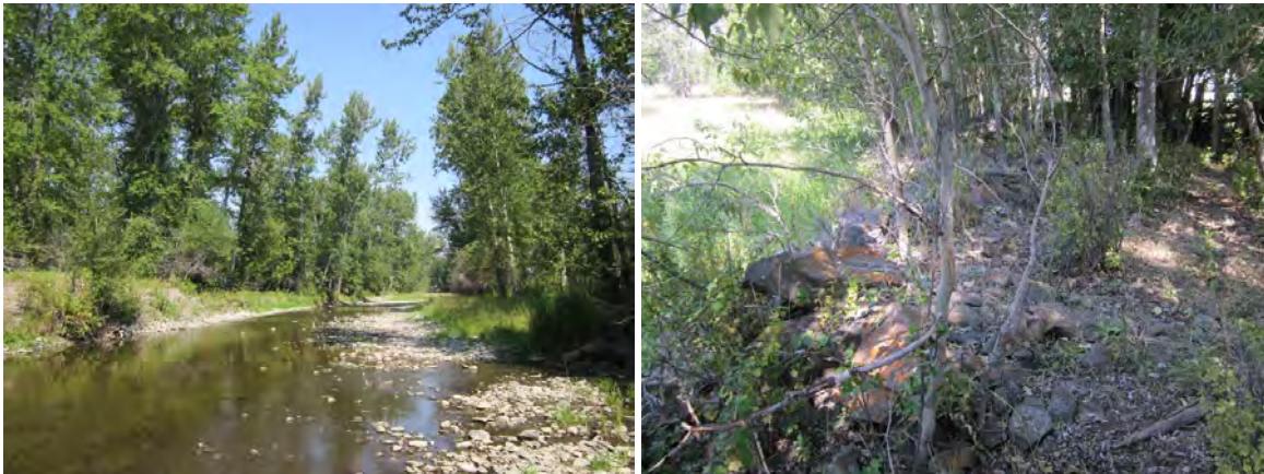
FIGURE 96. TYPICAL VIEW OF PROPERTY 2 (L) AND OLD RIPRAP THAT WAS NO LONGER NEAR THE CHANNEL.
