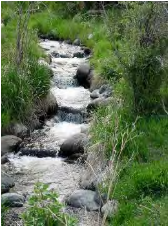
FIGURE 60. STEP/POOL SEQUENCE CONSTRUCTED UPSTREAM OF THE CULVERT DIVERTING NORTH FORK FRIDLEY CREEK UNDER THE PARK BRANCH CANAL, TO MATCH PRE-PROJECT GRADE AND PROVIDE FISH PASSAGE FROM THE YELLOWSTONE RIVER.
