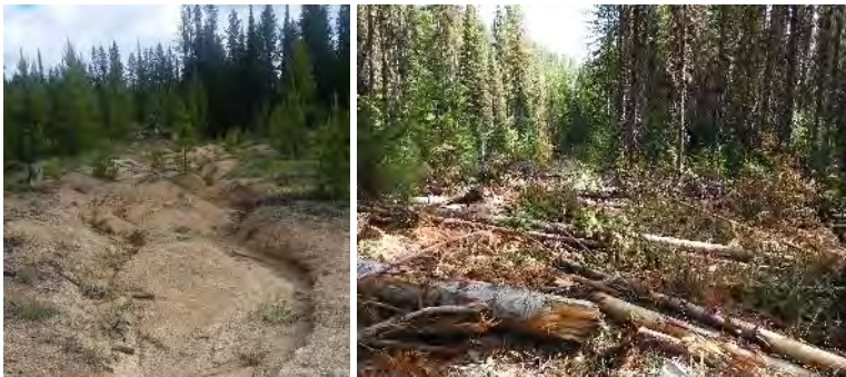
FIGURE 17. GRANITE CREEK CULVERT REMOVAL AND FISH PASSAGE BEFORE (L) AND AFTER (R).
