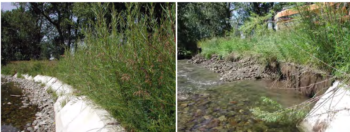
FIGURE 83. STABILIZED BANK ON THE SHIELDS RIVER (L) AND REMOVAL OF CONCRETE BLOCK AND INSTALLATION OF ROCK TOE (R).
