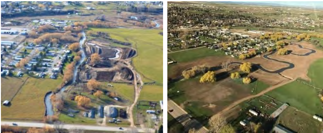
FIGURE 21. BIG SPRING CREEK DURING CONSTRUCTION (L, ORIGINAL CHANNEL) AND POST CONSTRUCTION (R, 2017).
