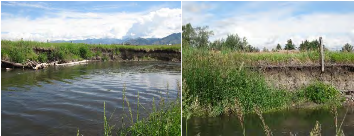
FIGURE 54. BANK 3 ON THE EAST GALLATIN RIVER BANK RESTORATION PROJECT (L) AND VERTICAL EXPOSED STREAM BANK AND EVIDENCE OF LATERAL MOVEMENT, AS INDICATED BY THE HANGING FENCE POST (R).
