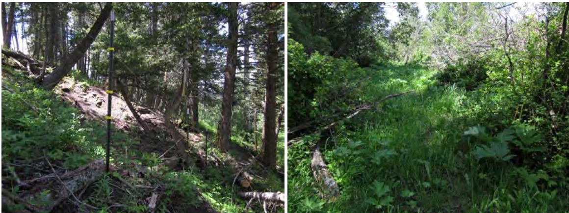
FIGURE 68. NEW FENCE INSTALLED TO PREVENT LIVESTOCK FROM ACCESSING NORTH FORK HORSE CREEK FROM BENCH (L) AND TYPICAL VIEW OF THE FENCED OFF HILL SLOPE PROTECTED BY FENCING INSTALLED ALONG THE TOP OF THE BENCH (R).
