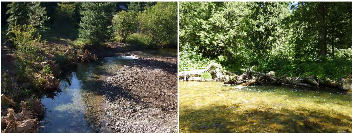
FIGURE 128. EAST FORK BULL RIVER CHANNEL STABILIZATION AFTER CONSTRUCTION (L) AND IN 2017 (R).
