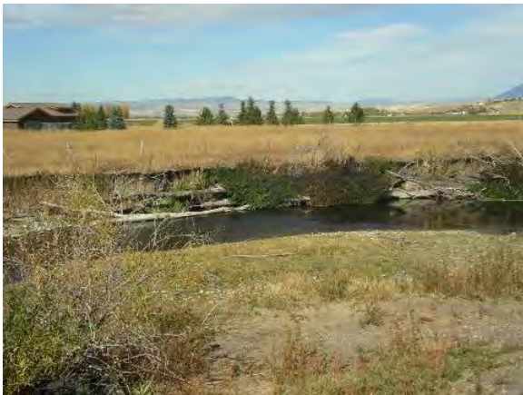
FIGURE 47. BANK 3 ON THE EAST GALLATIN RIVER, SHOWING CABLED-IN COTTONWOODS THAT WERE PART OF AN EARLIER BANK STABILIZATION EFFORT.
