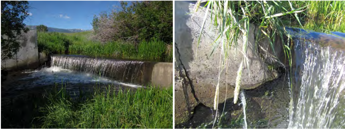
FIGURE 108. THE THIEL CREEK FISH BARRIER (L) AND CRUMBLING CONCRETE ON THE RIGHT SIDE OF THE BARRIER (R).
