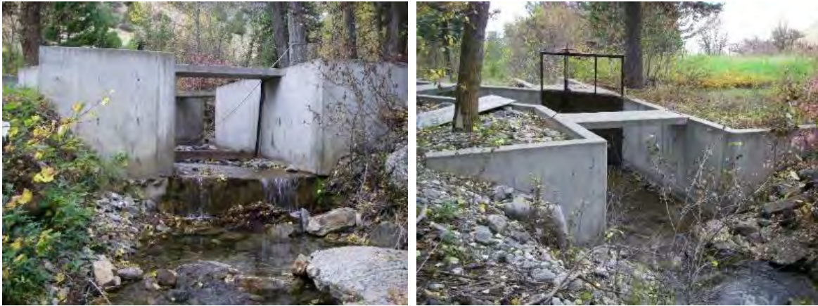
FIGURE 22. BOSTWICK CREEK FISH BARRIER BEFORE (L) AND AFTER MODIFICATION (R).
