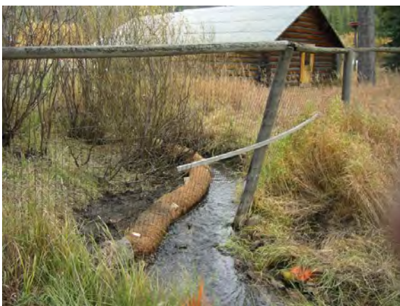
FIGURE 115. NEW BANK BUILT WITH STRAW WATTLE AND BACK FILLED WITH SEDIMENT EXCAVATED FROM CHANNEL.
