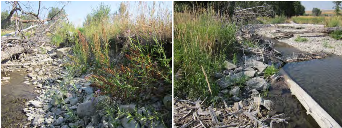
FIGURE 85. STREAM BANK POTENTIALLY BEING THE RESTORED BANK (L) AND BANK ARMORING AND LARGE WOODY DEBRIS (R)
