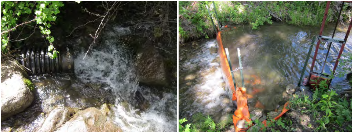
FIGURE 76. BYPASS PIPE (L) AND CHECK BOARDS IMPOUNDING FLOWS TO DELIVER WATER TO THE HEAD GATE (R).
