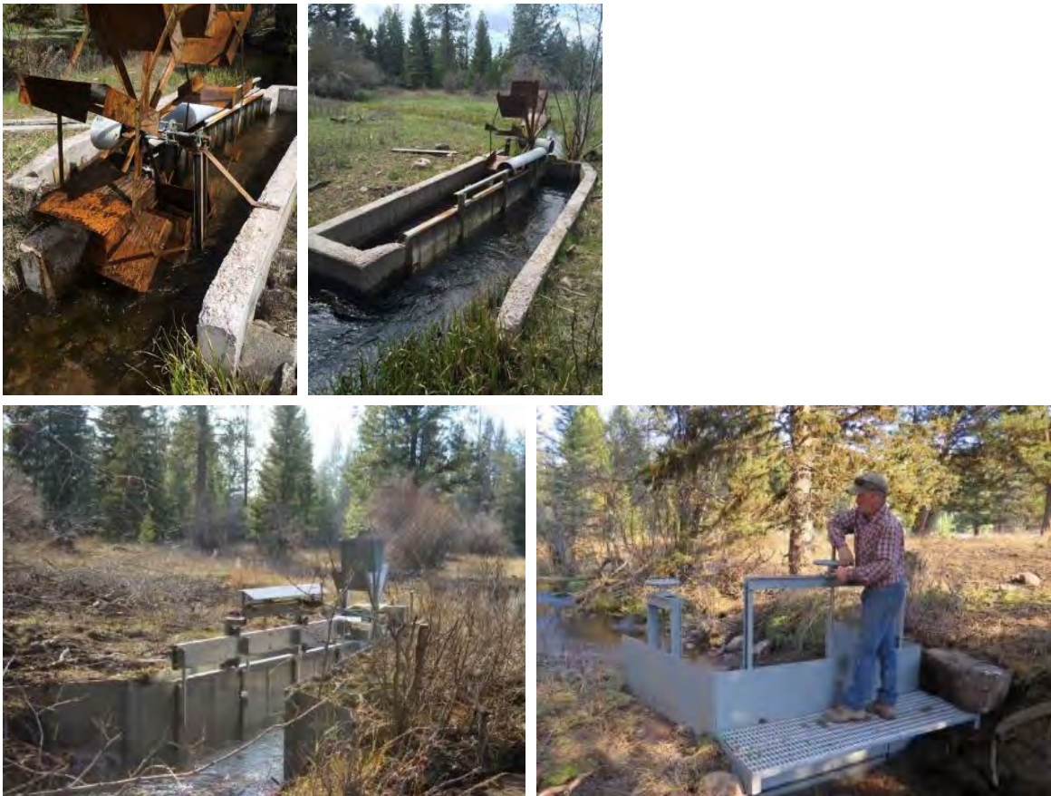
FIGURE 35. OLD, NON-FUNCTIONAL FISH SCREEN (TOP) AND NEWLY INSTALLED SCREEN AND HEADGATE (BOTTOM).
