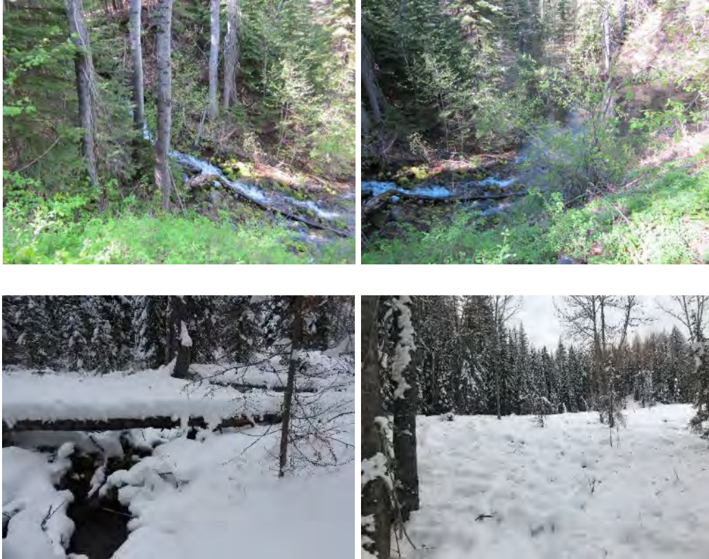
FIGURE 30. MARTINA CREEK; BEFORE CONSTRUCTION, THE STREAM WAS DIVERTED INTO A DREDGE POND (TOP) AND AFTER CONSTRUCTION THE STREAM WAS RETURNED TO ITS CHANNEL (BOTTOM L), WITH THE POND FILLED (BOTTOM R).
