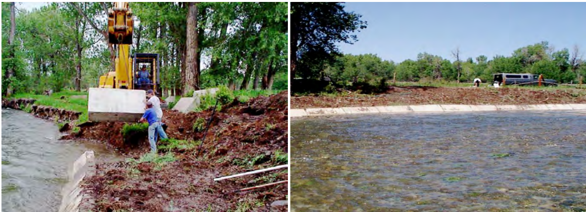
FIGURE 82. PROJECT CONSTRUCTION PHOTO SHOWING EXISTING ERODING BANK (L) AND CONCRETE BLOCKS INSTALLED ALONG THE BANK LINE (R).
