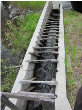
FIGURE 102. DENIL FISH LADDER ON SOUTH FORK FRIDLEY CREEK.
