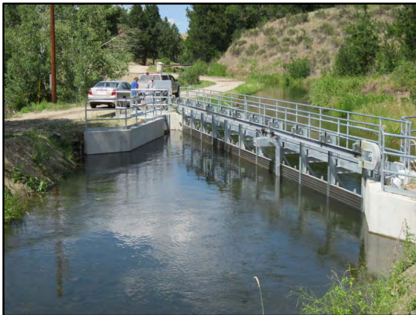
Photo Illustration 2. Fish screens installed into irrigation canals to prevent fish from being lost down the ditches. The upper photo shows a fish screen installed into an irrigation diversion located on the Blackfoot River near the town of Lincoln in Lewis and Clark County. This screen prevents westslope cutthroat trout, bull trout, brown trout, mountain whitefish and native suckers from being entrained into the ditch. The lower photo shows a fish screen installed into the Hedge Canal, a large diversion located on the Bitterroot River near Hamilton in Ravalli County. This screen prevents westslope cutthroat trout, bull trout, rainbow trout, brown trout, mountain whitefish and native non-game fish from being entrained into the canal.
