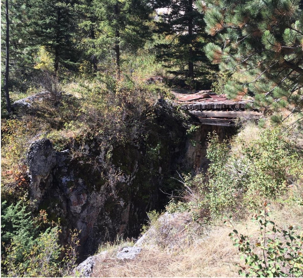
Figure 13: The failing Tiger Creek Trestle along the Belt Creek Railway (24CA1315) in Sluice Boxes State Park.
