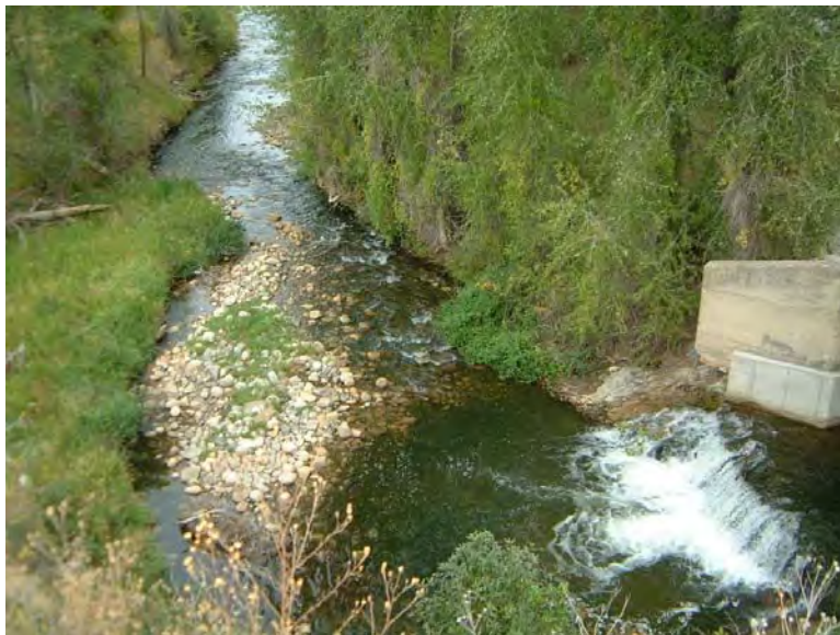
FIGURE 19. IMPASSIBLE CULVERT ON CLEAR CREEK.
