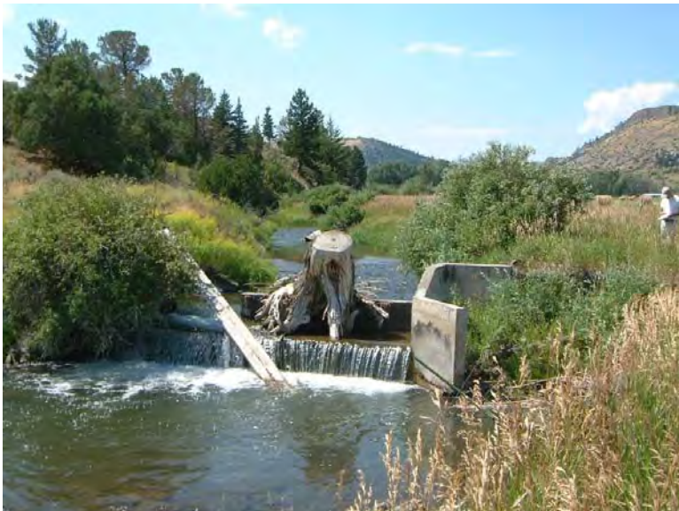
FIGURE 13. IRRIGATION DIVERSION BLOCKING FISH PASSAGE ON BRACKETT CREEK (2003).
