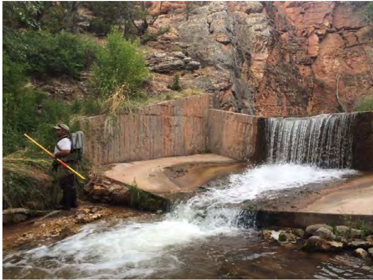
FIGURE 26. DOWNSTREAM END OF APRON SHOWING LACK OF A PLUNGE POOL.
