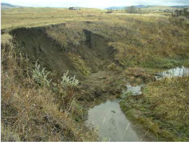
FIGURE 52. EXAMPLE OF AN ERODING TERRACE ON FLESHMAN CREEK WITHIN THE PROJECT AREA.
