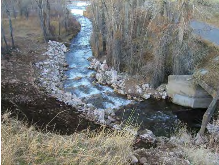
FIGURE 20. POST-CONSTRUCTION PHOTO OF STEP-POOL SEQUENCE PROVIDING PASSAGE UP TO, AND THROUGH, THE
