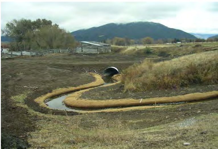
FIGURE 53. EXAMPLE OF NEWLY CONSTRUCTED CHANNEL ON FLESHMAN CREEK AND STREAM CROSSING WITH BOTTOMLESS ARCH CULVERT AND OVERFLOW PIPES.
