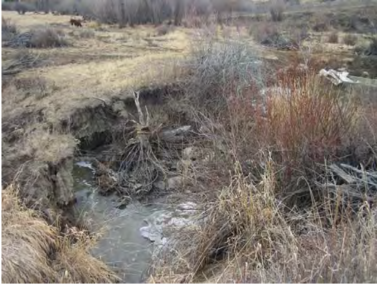
FIGURE 30. EXAMPLE OF CHANNEL DOWN-CUTTING, AND A VERTICAL BANK SLATED FOR SLOPING.
