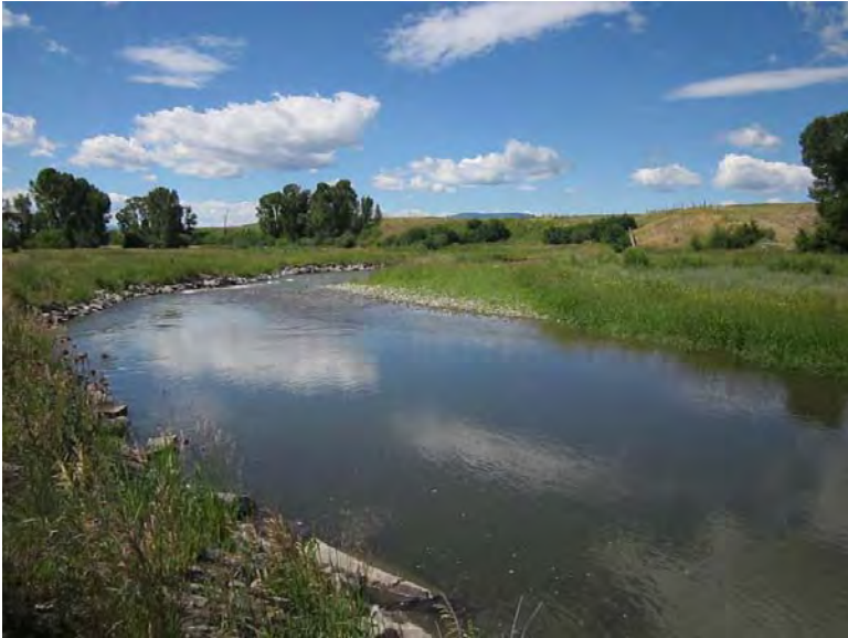
FIGURE 83. EXAMPLE OF BANK STABILIZATION ON THE SHIELDS RIVER AFTER FAILURE OF THE ROOT WADS AND TREE REVETMENTS.
