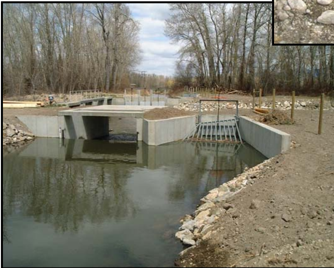
Photo Illustration 9. Installation of a large siphon located underneath Skalkaho Creek at the Hedge Canal crossing near Hamilton. Skalkaho Creek is a significant tributary to the Bitterroot River. The installed siphon separates canal water from creek water and prevents the loss of fish into the large irrigation system. The upper photo shows the Hedge Canal (foreground) entering into and intermingling with Skalkaho Creek prior to the installation of the siphon. The middle photo shows the construction of the siphon inlet works. The lower photo shows the completed siphon (without the controlling headgate installed). This project benefits both westslope cutthroat trout and bull trout.
