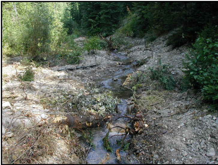
Photo Illustration 6. Channel restoration on Eustache Creek, a tributary to Ninemile Creek in the Clark Fork watershed. Historical placer mining in the Eustache drainage created a braided and intermittent stream channel (upper photo). Installation of a series of ground water retention sills (middle photo) resulted in the establishment of a permanently flowing stream channel (lower photo), benefiting both westslope cutthroat trout and bull trout. Photos provided by the USFS.
