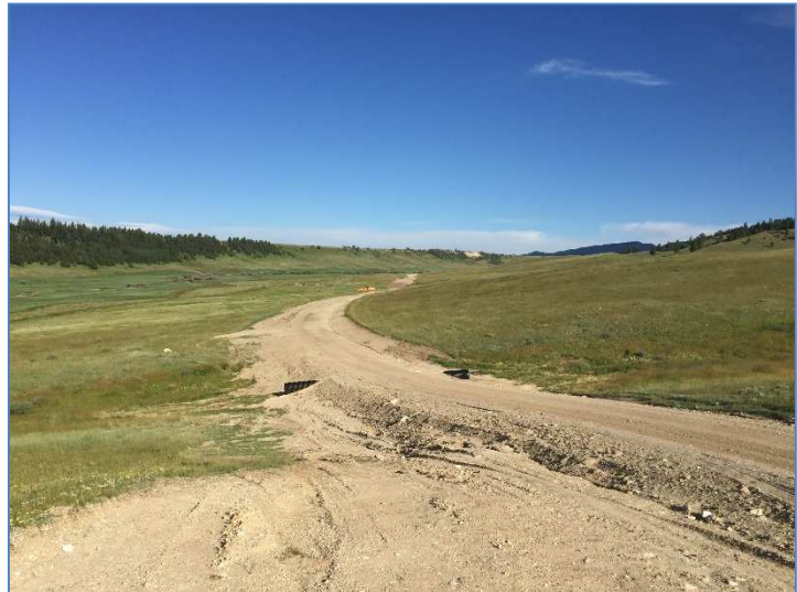
Access road improvements constructed during 2017 at Haymaker WMA, Wheatland County (Photo Credit: T. Mannat).
